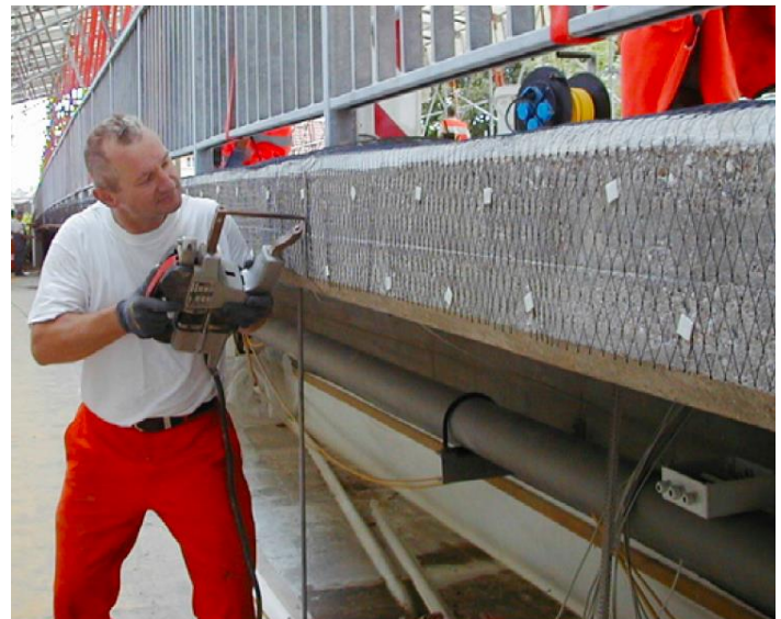
Abb. 2: Application of a titanium grid anode (to be covered by mortar). Source: suicorr AG
